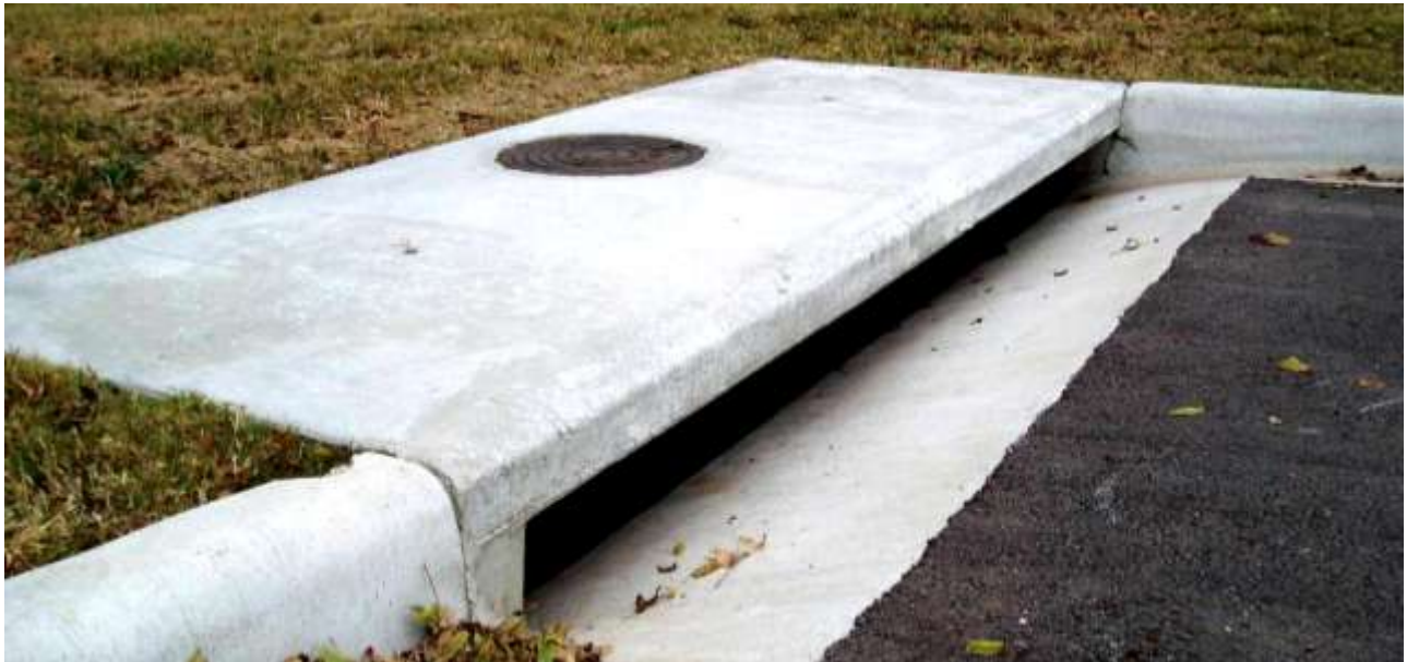
Figure 7.2. Storm drain in Kyle adjacent to Steeplechase Park. Stormwater engineering analyses are an important initial part of the urban management strategy.
