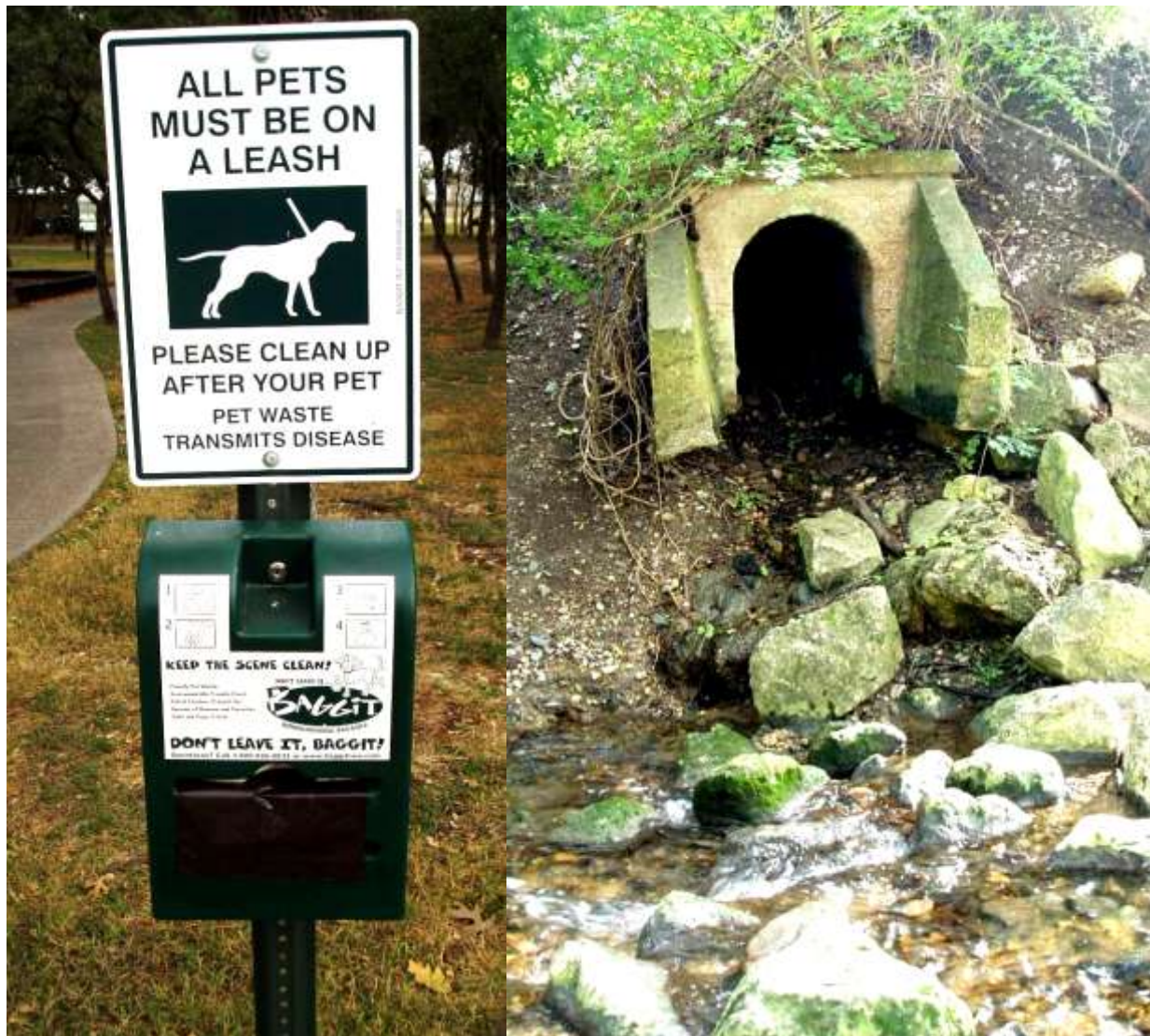
Figure 7.3. Pet waste station in Plum Creek community and storm drain outlet in Lockhart City Park. Management of pet waste and stormwater are important activities in urbanized areas of the watershed.
